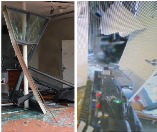
Fig. 7. The damaged front of the building that the robot needed to enter (left). In addition to clearing or stabilising this debris, the robot also needed to negotiate a doorway that was partially obstructed with low hanging obstacles (right). This view from the wide angle camera mounted to the robot's existing pan-tilt-zoom camera affords a view of the robot, in context among these obstacles, something that would require lengthy continuous scanning with a traditional narrow angle camera. Note that the left and right edges have been substantially cropped for reasons of operational sensitivity; the lower left frame of Figure 6 is representative of the field of view of this camera.
